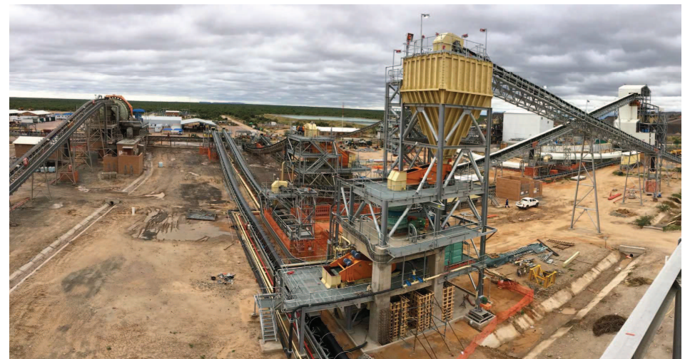
Tertiary crusher with XRT building in the background
